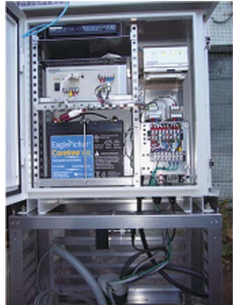
Fig. 8. External view of the above-ground part of an observatory. From top left to bottom left: ISDN router, power source controller, and accumulator. From top right to bottom right: observation controller and arrester terminal block.
